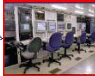
Ground Control Station System
